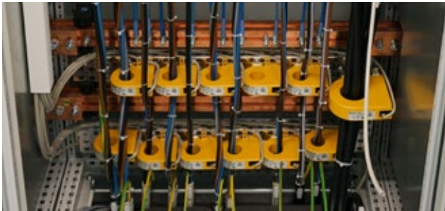
Residual current monitoring of final circuits and outgoing circuits
