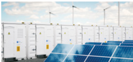
Battery energy storage systems (BESS)
